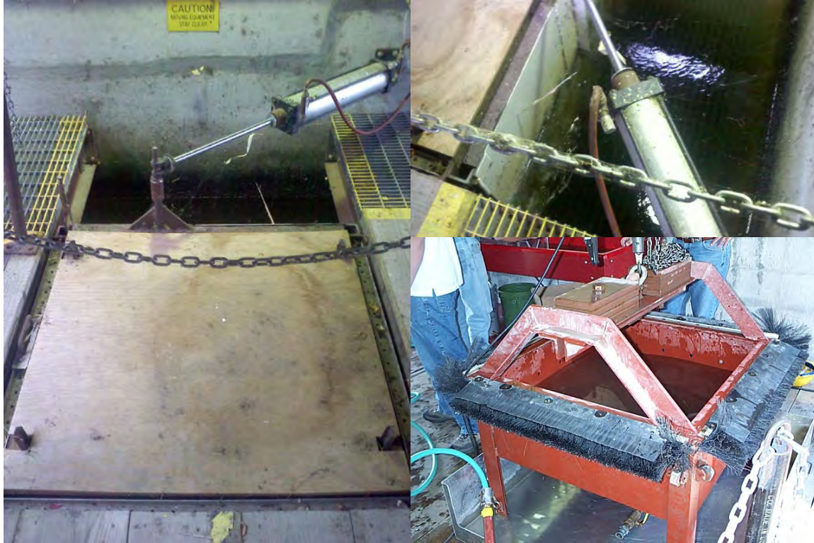
Figure 2. Adult trapping facility at Rocky Reach Dam. The pneumatic arm (left and top right) activates a gate that guides fish into a holding vessel (bottom right, shown lifted). Trapped fish are either allowed to exit the holding vessel by opening the gate, or are lifted for processing.
