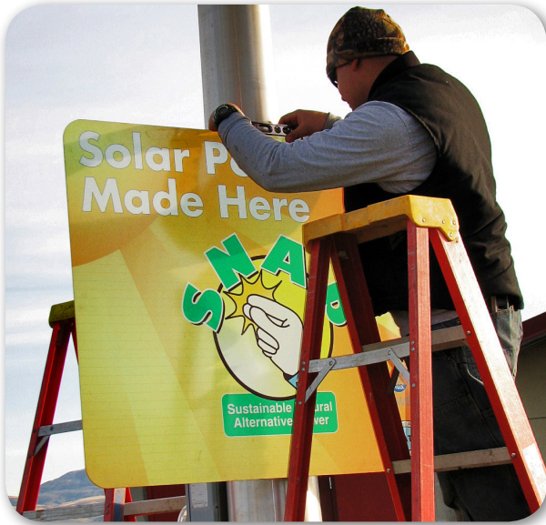
Above: J.C. Ellis of McCandlish Electric secures the new sign on the solar array at Pioneer Middle School.
