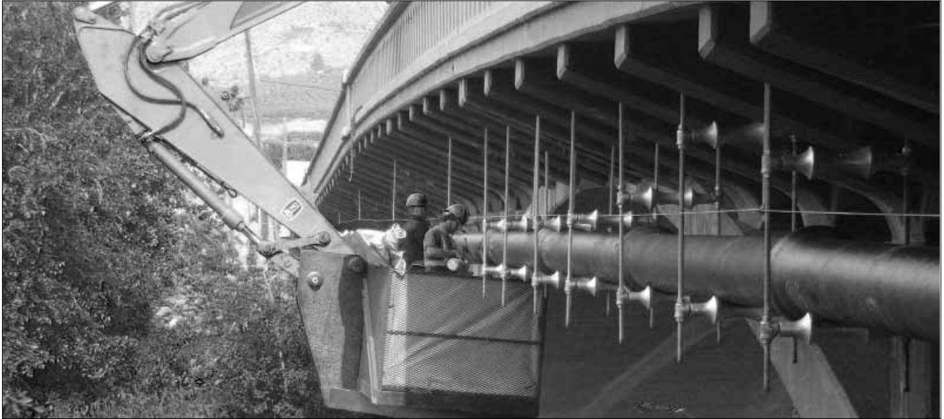
Contractors install water pipe under the Monitor Bridge – the most difficult part of the PUD project to bring water to the community
