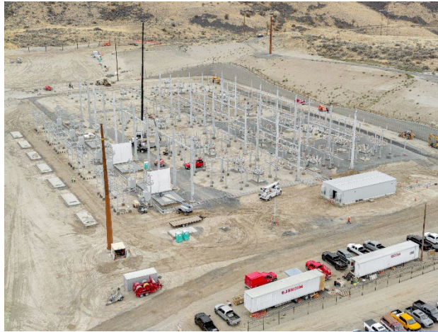
Jumpoff Ridge Switchyard 2025
