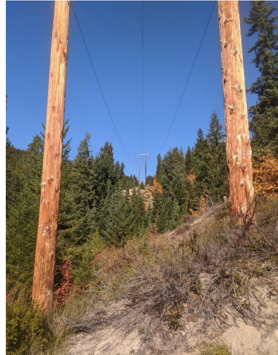
Upper Valley Transmission 2024-2028
