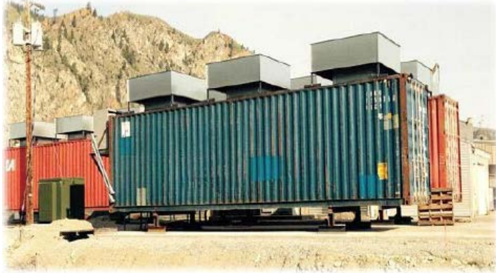
Cargo containers converted to data mining rigs.
