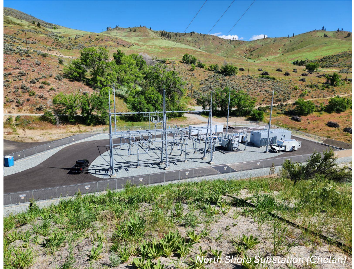
North Shore Substation (Chelan)
